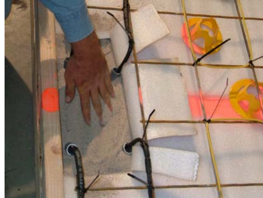
6. Once the jumper is complete, fill in the exposed area with sand so that conduit is completely covered.
