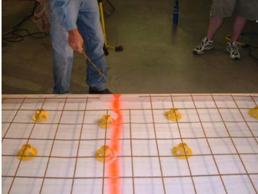
1. After insulation, castle chairs and welded wire fabric have been installed, use spray paint to indicate where any joint (expansion, mark, strike, etc) will be located.
